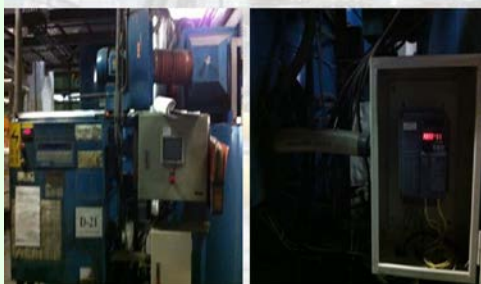
酯粒乾燥機Process Blower加裝Inverter
